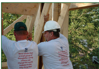
Below: Royal Roofing Company President-Dan Davis (right) with Royal Employee-Joel Trombley working on Royal sponsored home.
