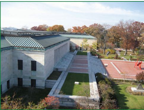
Photo Above: An elongated view of the Toledo Museum of Art—"Main building"; pre re-roof state.
